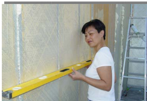
Ms. No, project manager, said walls are stronger, straighter and more energy efficient.
